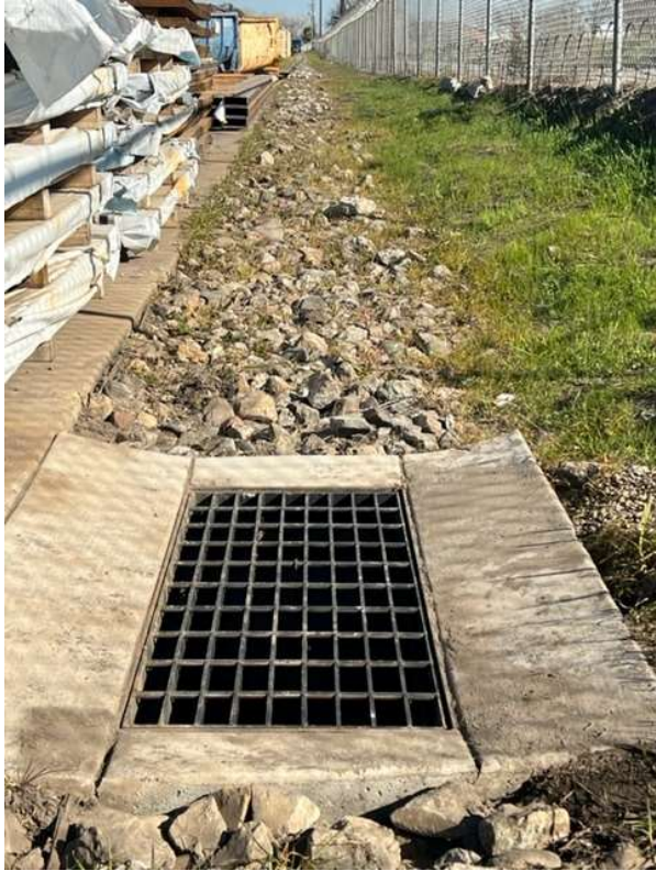
South Infiltration Trench
