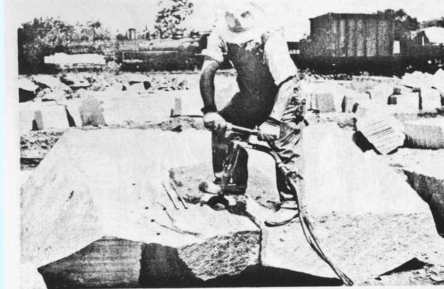
FIGURE 8. Modern wet drilling with jackhammer in plug yard. Rubber cup prevents spraying operator with water. (Courtesy of Rock of Ages.)
