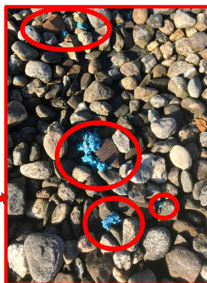
PFAS Residue in Roof Ballast from Chunking of Coating Agglomeration Occurring in Stacks ≤13,000,000 ng/Kg PFOA
