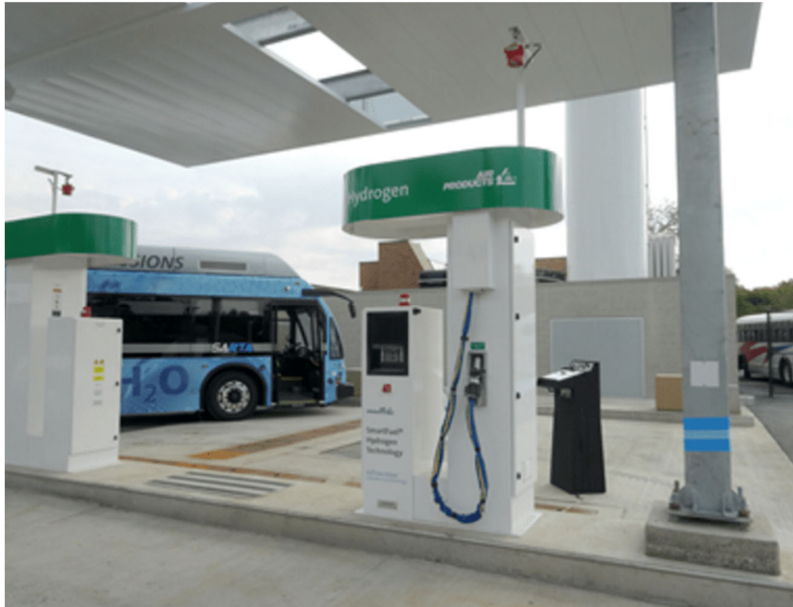
SARTA Hydrogen Fuel Cell Bus Refueling Station
