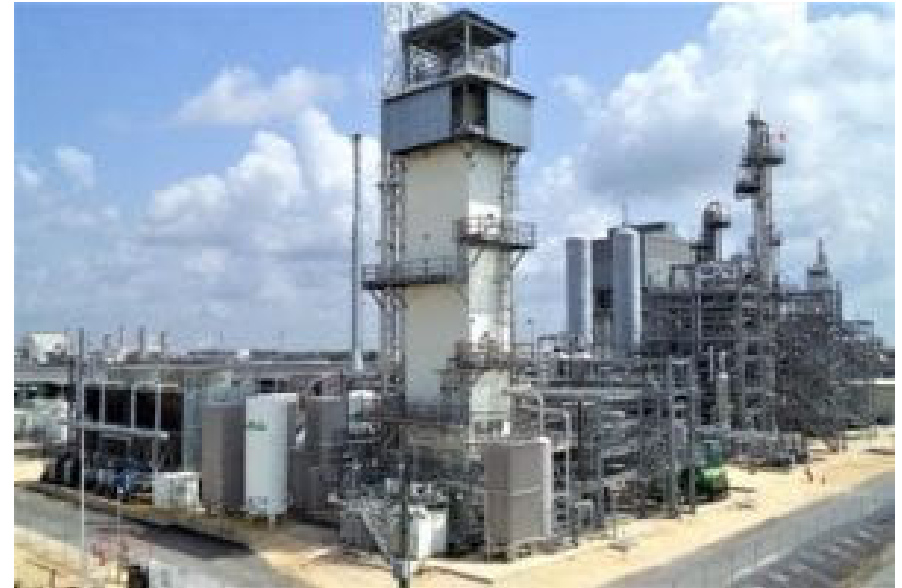
50 MMSCFD (120,000 kg/d) capacity Steam Methane Reformer Air Products Geismar, LA
