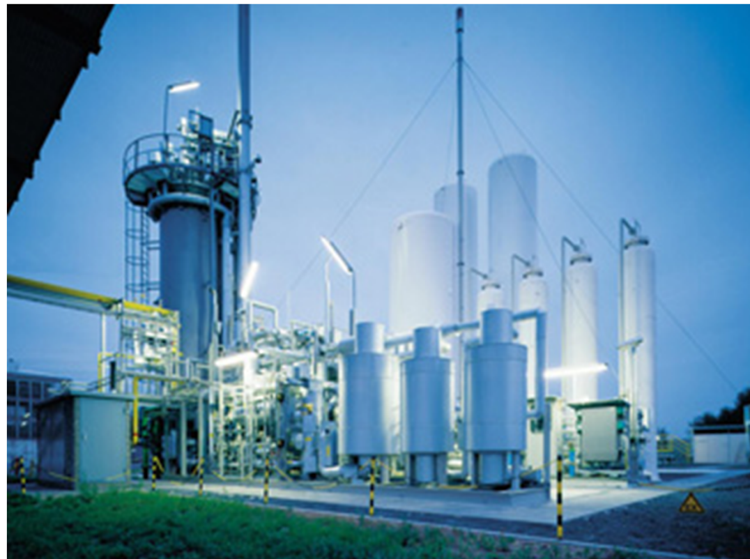
Steam Methane Reformer
