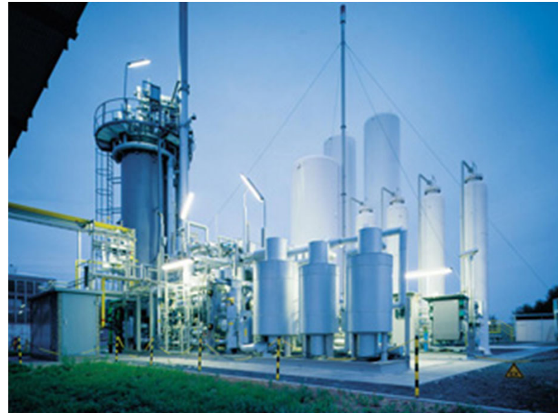
Steam Methane Reformer
