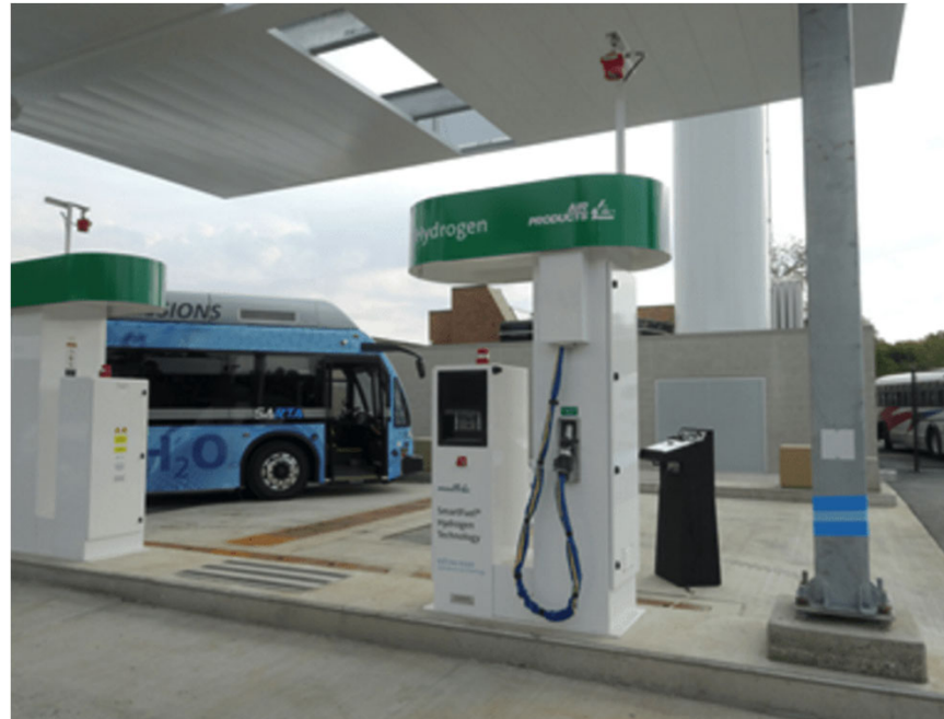
H2 Refueling Station Stark Area Regional Transit Authority Canton, Ohio
