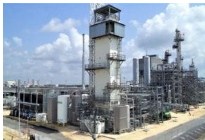
50 MMSCFD (120,000 kg/d) capacity Steam Methane Reformer Air Products Geismar, LA
