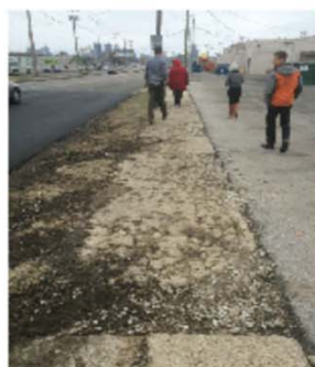
Sidewalk on Mound crumbling
